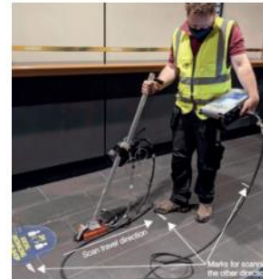
High-frequency impulse radar (up to 0.50m depth) to scan reinforcement in concrete slab of 32 NR.
