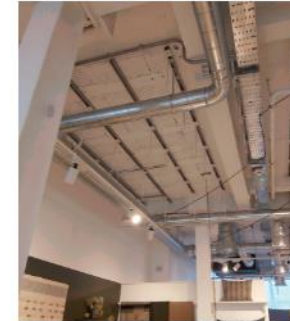
34 North Row. The structure is generally exposed. The semi-exposed first floor visible from ground floor.
