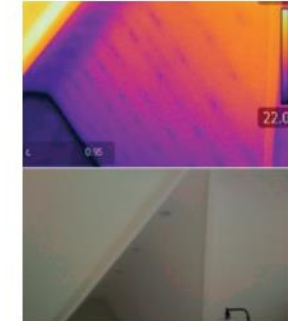
31-33 North Row. The structure is generally hidden behind the finishes. Thermal camera identified the rafter locations & spacing.
